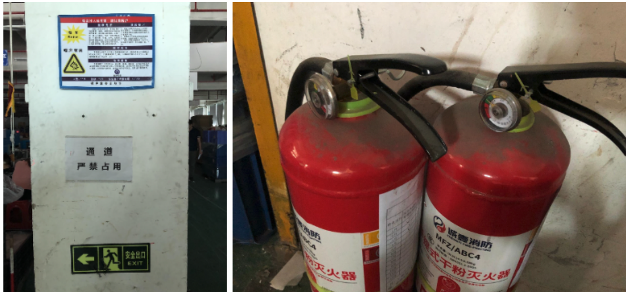
(Left: Emergency exit sign. Right: Fire extinguishers)
